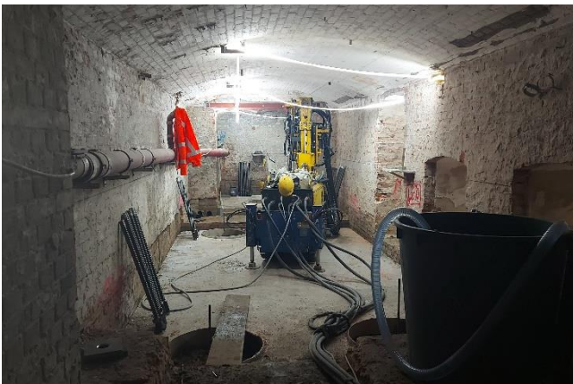
(2) The working conditions in the basement of the Märkisches Museum were highly confined with a room height of 2.6 m.
