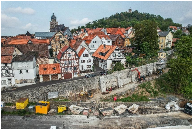
(1) The wall of the German town Homberg was extensively rehabilitated over a length of 100 m.
