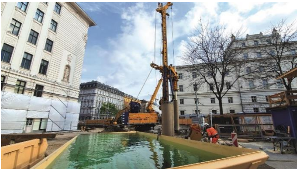
(2) A BAUER BG 39 was used for the contract section U5/2 “Frankhplatz Nord” shaft.
