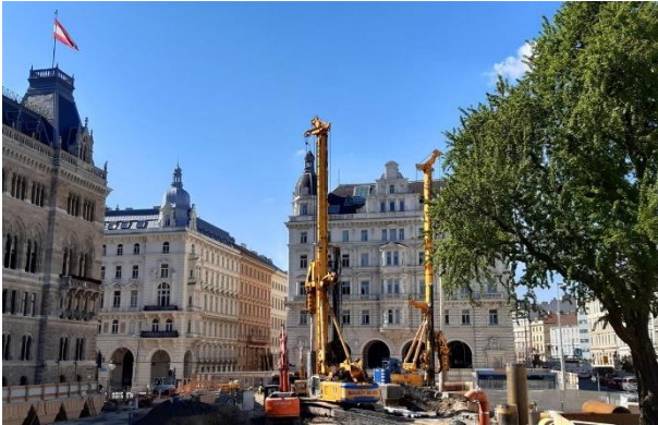
(1) A BAUER BG 45 and a BG 40 during drilling work for the U2/22 “Friedrich-Schmidt-Platz” shaft.
