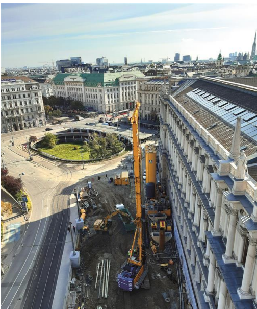
(3) A BAUER BG 45 was in operation at the section U2/22 “Schottentor” connecting structure.
